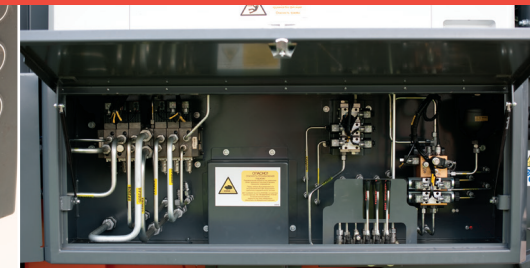
Steel pipework for better heat dissipation
