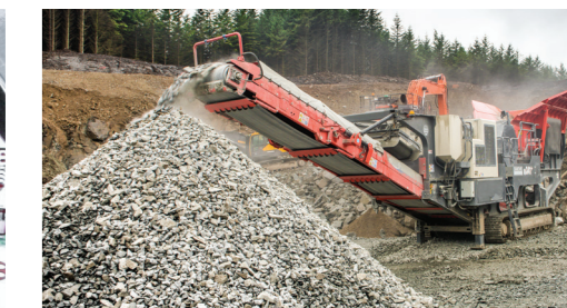
Long main conveyor for massive stockpiling
