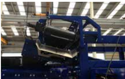
Overband Magnet- fitted to collection conveyor to extract ferrous metal
